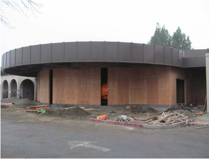
East 14 th Street - East side (front), Automated Materials Handling area.
