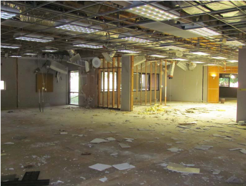
East 14 th Street - early demolition. Looking toward staff offices and Hughes room.
