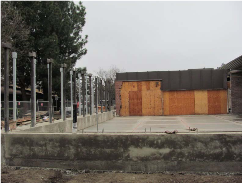
East 14 th Street - West side Children's area expansion, new cement slab and wall framing, view 1.
