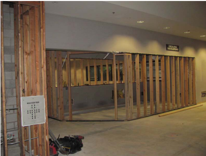
East 14 th Street - Early Construction, Branch Manager's Office in front of Hughes room.
