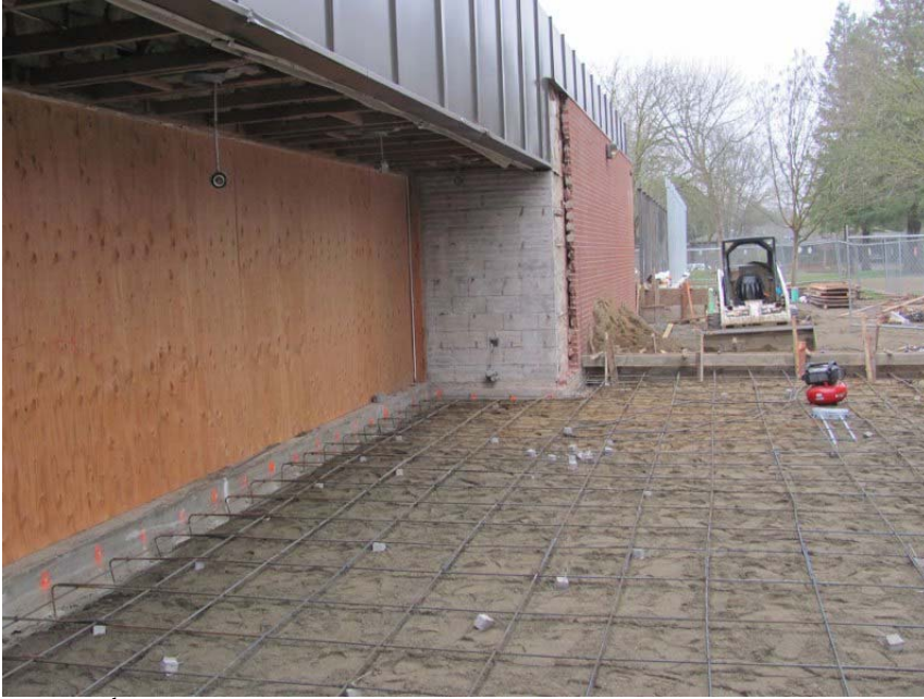
East 14 th Street - Reading garden area, getting ready for the cement slab.
