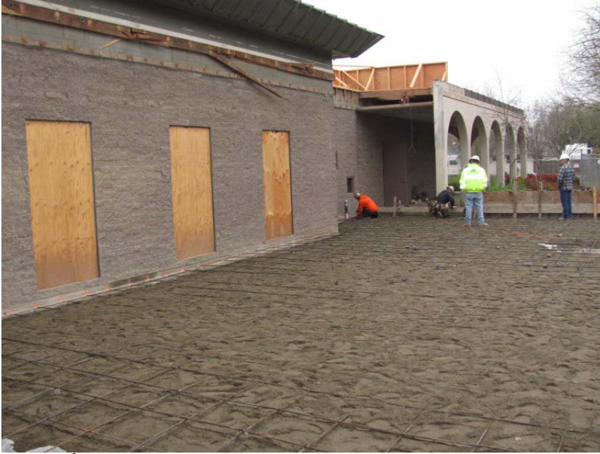
East 14 th Street - West side Children's area expansion, getting ready for the cement slab.
