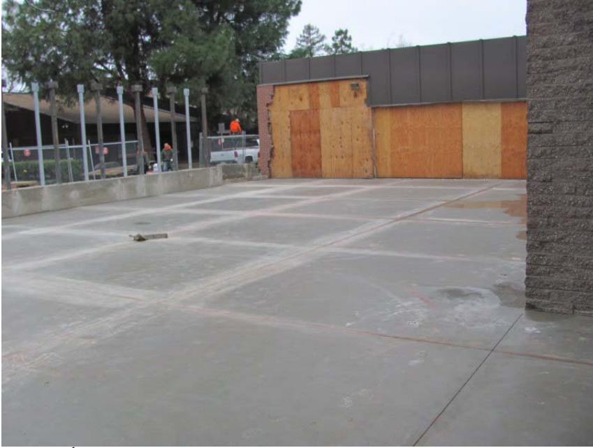
East 14 th Street - West side Children's area expansion, with new cement and wall framing, view 2.
