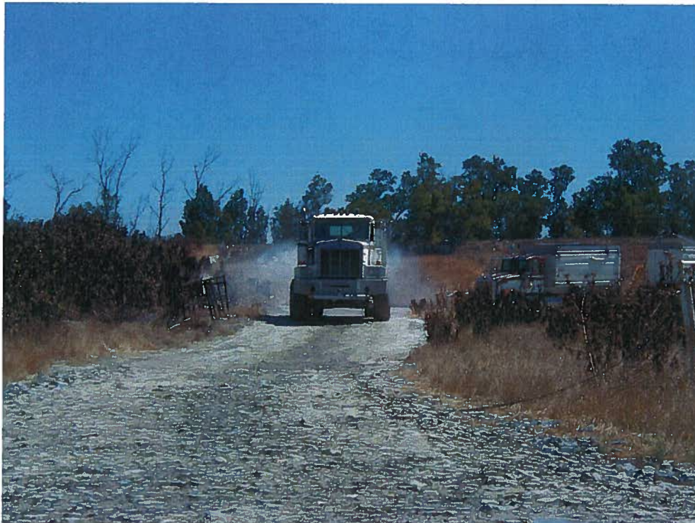
Water truck providing water to the project site access road and ingress/egress point at County Road 100B
