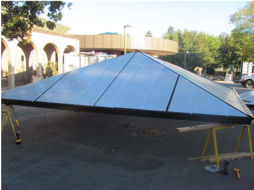
The skylights are being replaced, which will allow a great deal of natural light into the building.
