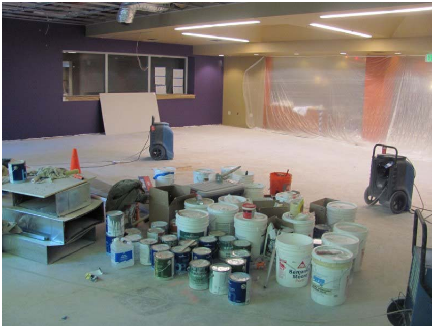
The Children's Room service desk can be seen beyond the plastic sheeting. Fiction and Non-Fiction books for older children will go in this room. The activities room is just behind us in this view. The Adult Fiction collection is beyond the window. Both this room and the activities room are new and are part of the expansion of the library
