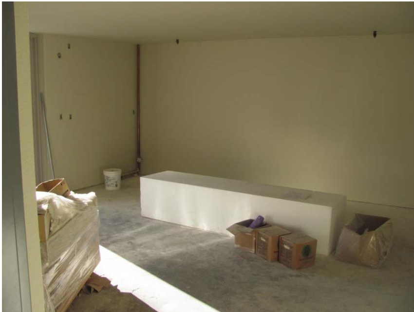
This is the work area set aside for the Friends of Davis Public Library. The items on the floor are for temporary construction storage.
