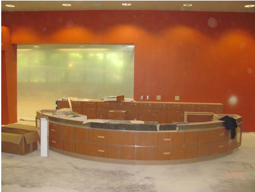
The Children's Room Service Desk is located centrally, with the new expansion area behind the plastic sheeting to the left.
