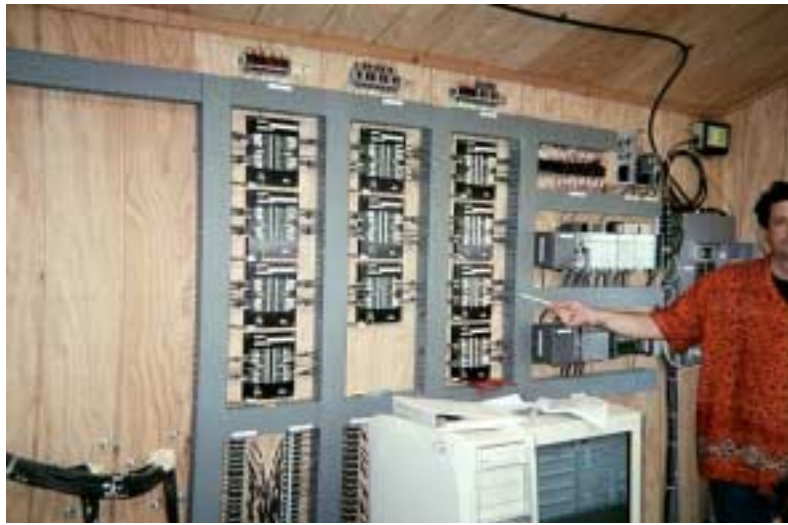
Image 4-1: Completed hardware installation
