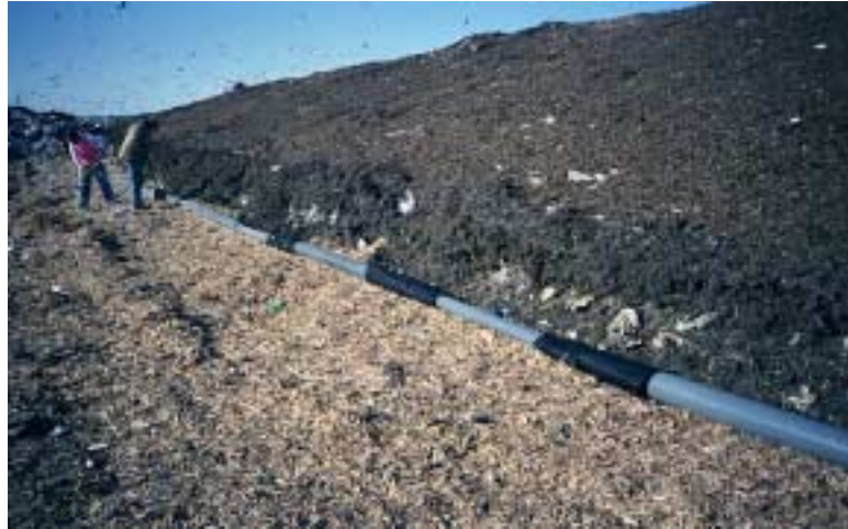
Image 3-2: Horizontal LFG collection line
