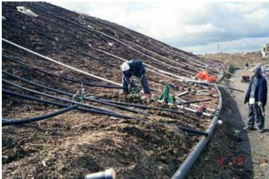
Image 13: Aerobic leachate injection header and lateral
