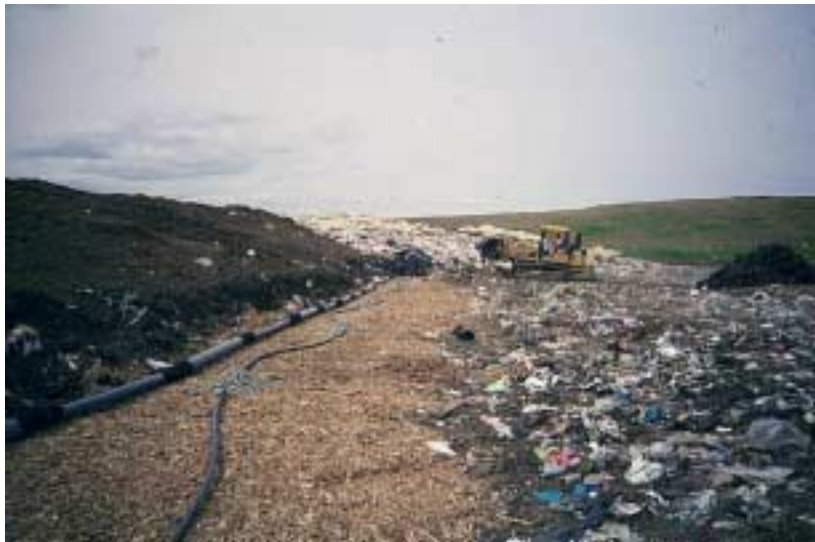
Image 1: Horizontal LFG and leachate injection lines installed and being covered by shredded tires.
