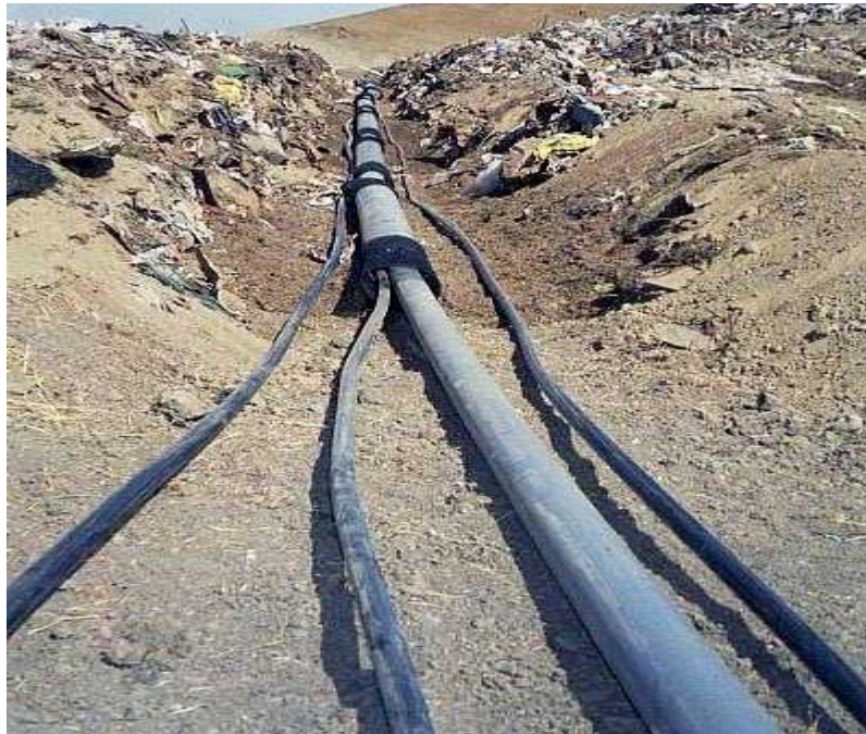
Image 10: Horizontal air collection line
