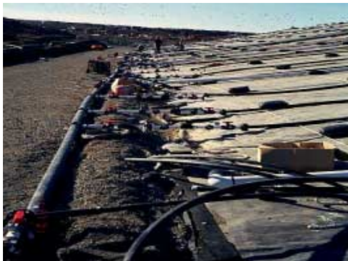
Image 6: Leachate injection header and laterals
