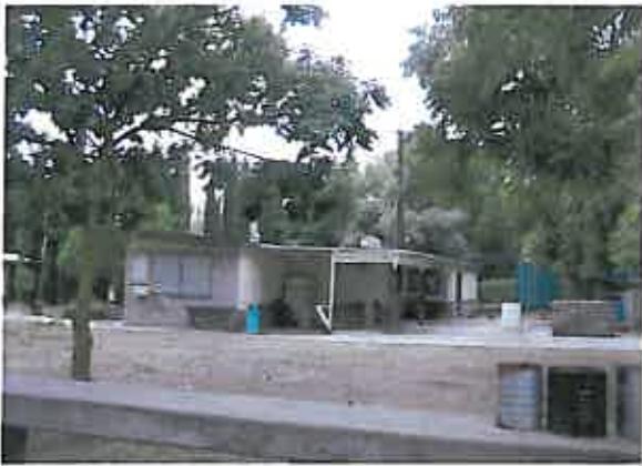
Figure 4: The existing restroom/kitchen structure is not code compliant and should eventually be replaced with a community facility.
