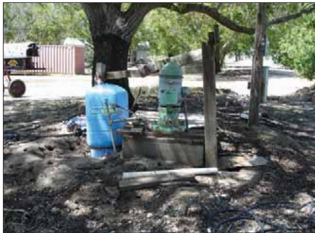
PHOTO 15: Domestic well located next to residence shown in Photo 19.
