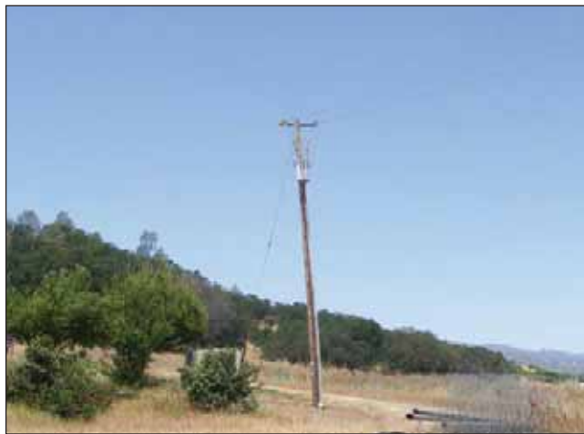
PHOTO 15: Power pole and associated transformer.
