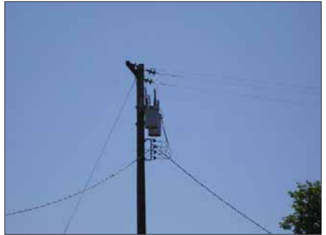
PHOTO 26: One of the pole-mounted transformers on Parcel 6.
