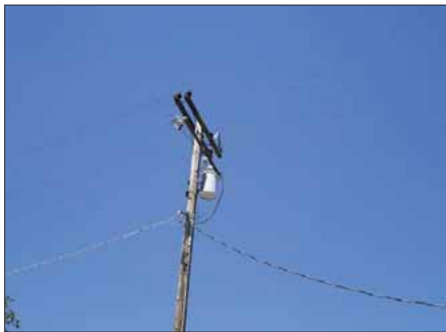
PHOTO 9: Pole mounted transformer on Parcel 2.
