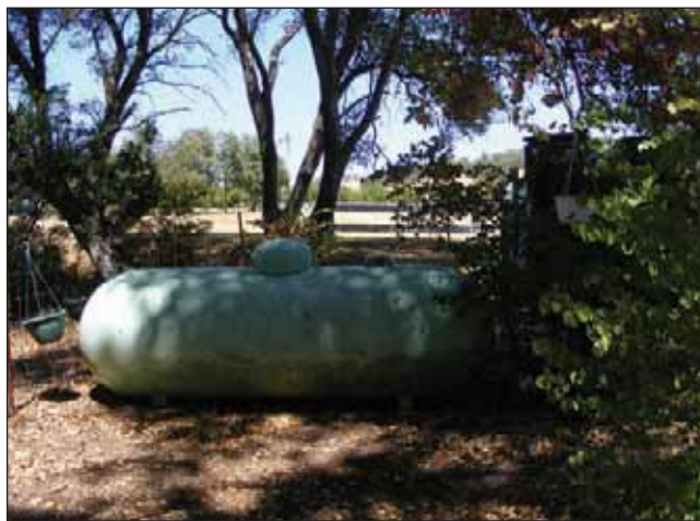
PHOTO 15: One approximately 5,000-gallon propane tank located behind the detached garage.
