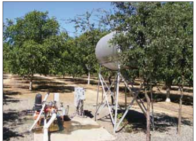
POTO 12: Electric pump next to one of the groves water well used to irrigate one of the orchards
