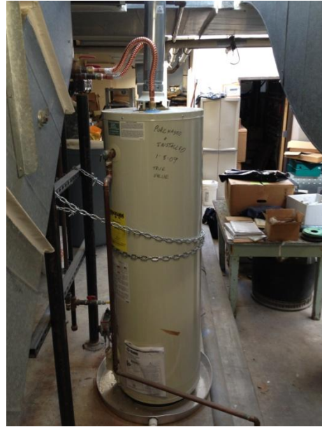
Image 86 – Domestic Hot Water Heater
