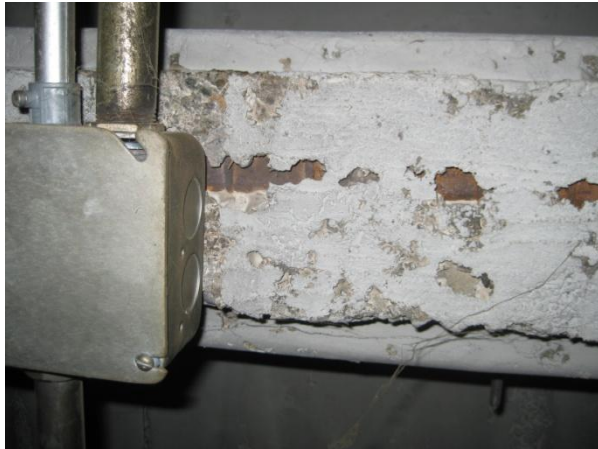
Image 73 – Exposed Rebar – Underside of Concrete Floor Joists
