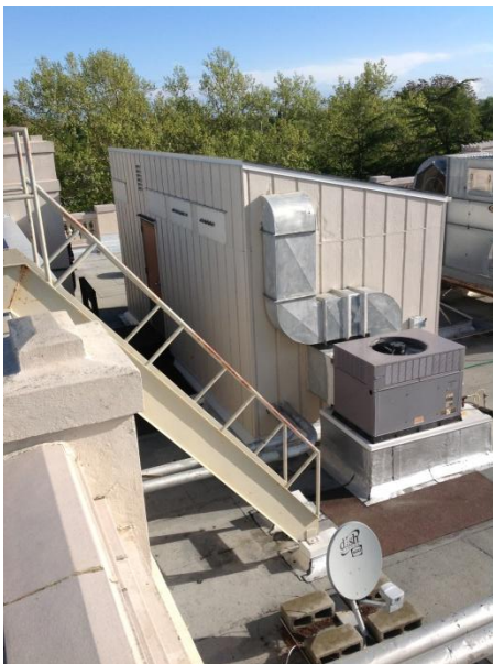
Image 35 – IT Room at Roof
