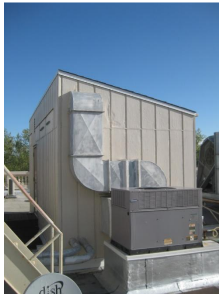
Image 36 – IT Room at Roof
