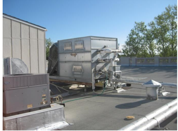
Image 38 – IT Room at Roof
