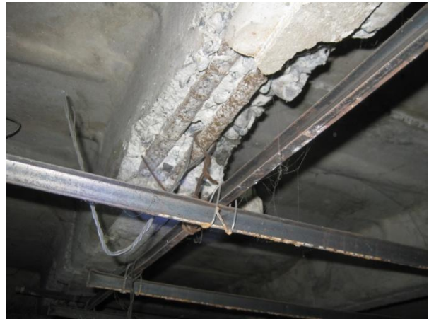
Image 80 – Exposed Rebar Supporting Ceiling Channels
