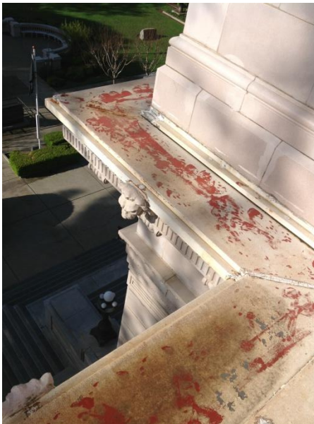
Image 27 – Standing Water at Cornice
