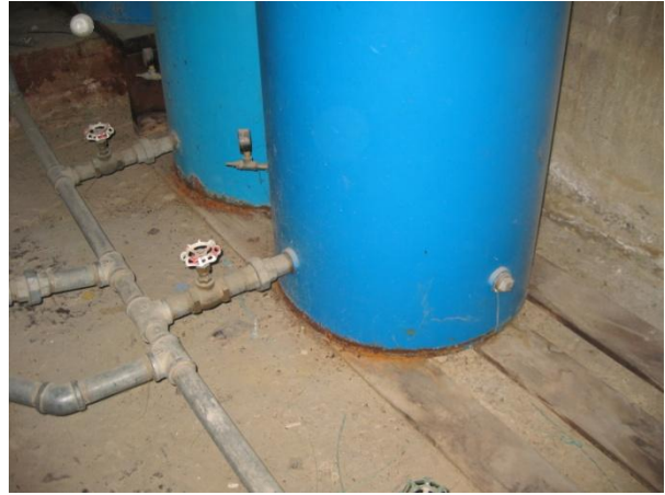
Image 78 – Tank without Base Anchorage
