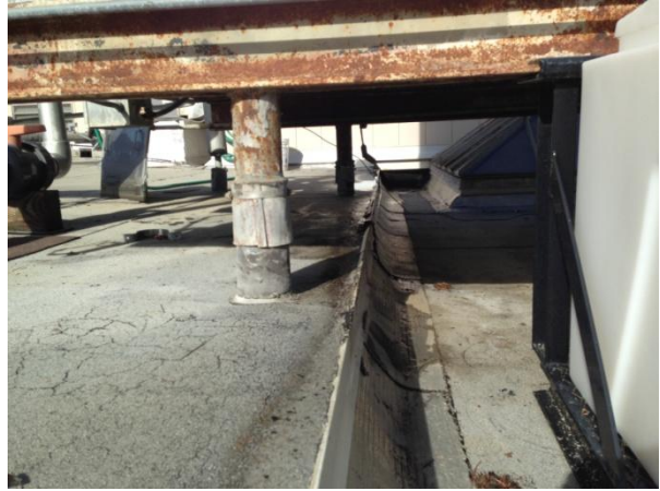
Image 42 – Fluid Cooler Leakage
