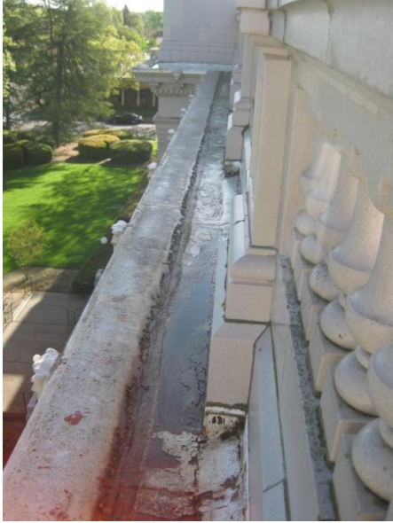
Image 29 – Standing Water at Cornice
