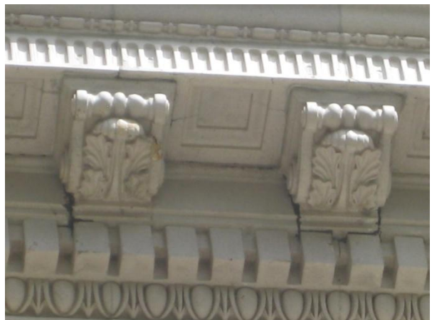
Image 20 – Water Damage at Underside of Cornice
