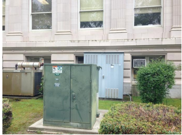
Image 26 – Transformer-Generator-Electrical Switch Gear
