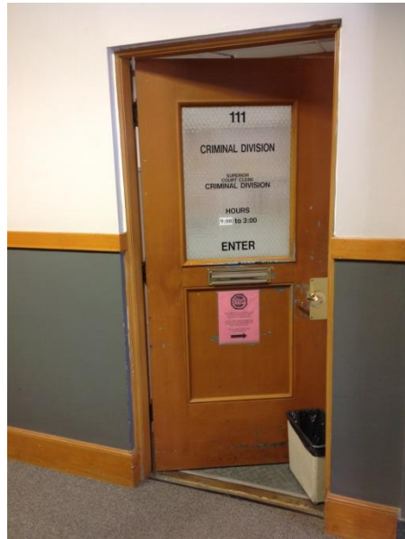
Image 68 – Finishes Worn at Door
