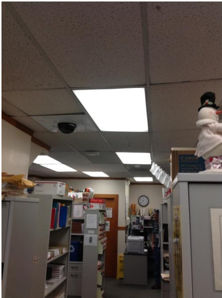
Image 67 – Damaged Ceiling Tile
