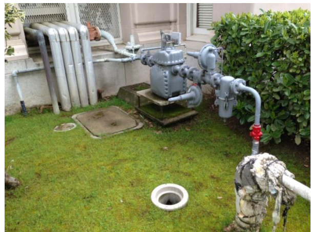
Image 24 – Plumbing Utility Entry – Domestic Water, Gas and Fire Sprinkler
