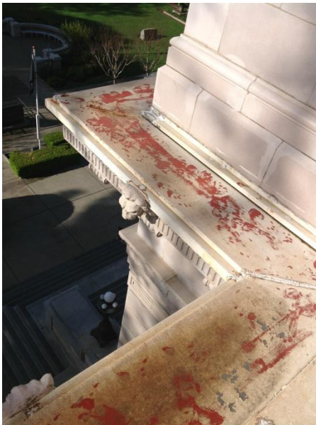
Image 27 – Standing Water at Cornice
