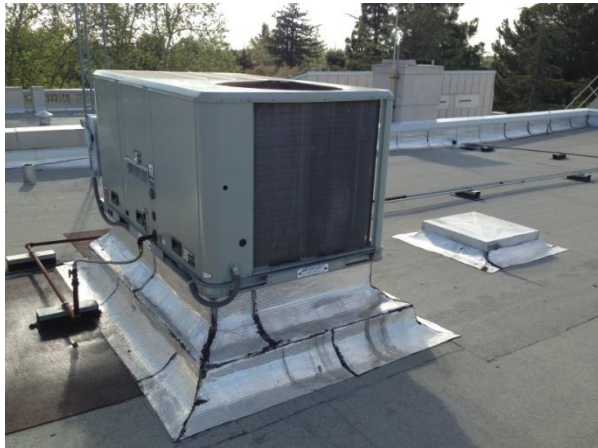
Image 43 – Fluid Cooler Mineral Deposit Build-up
