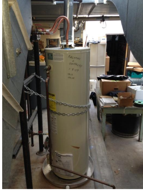
Image 86 – Domestic Hot Water Heater
