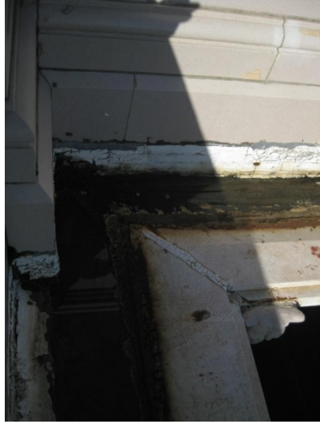
Image 30 – Standing Water at Cornice
