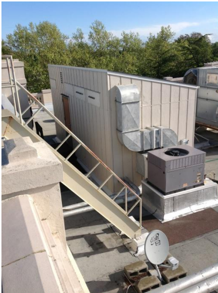
Image 35 – IT Room at Roof
