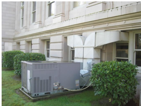
Image 23 – Mechanical Unit at Basement
