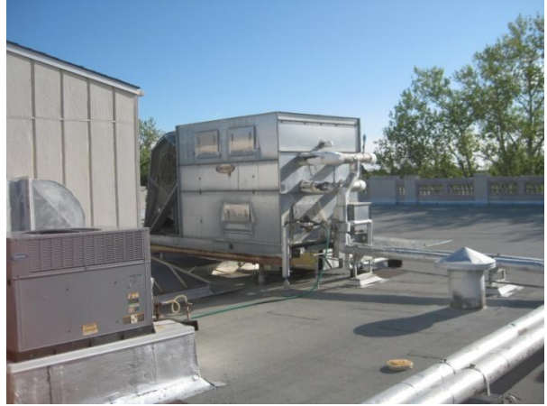
Image 38 – IT Room at Roof
