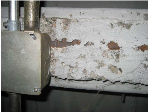
Image 73 – Exposed Rebar – Underside of Concrete Floor Joists
