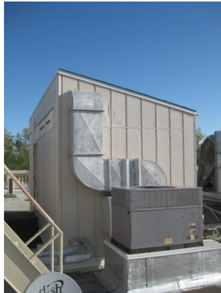
Image 36 – IT Room at Roof
