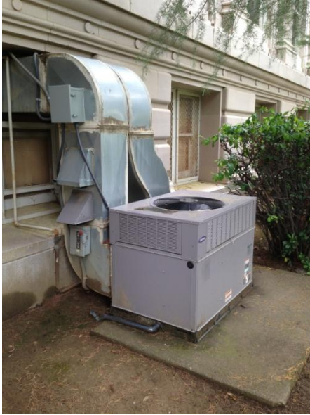
Image 25 – RAC at Grade – First Floor HVAC
