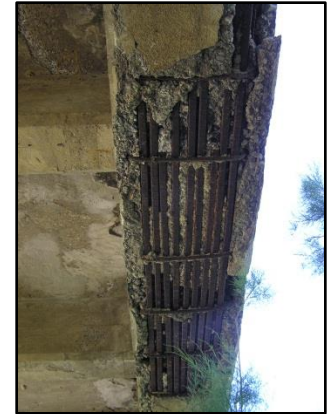
Severe Tie Girder Spalls
