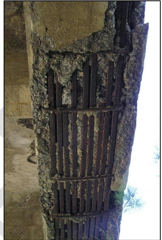
Rumsey Bridge Tie Girder Soffit Severely Spalled
