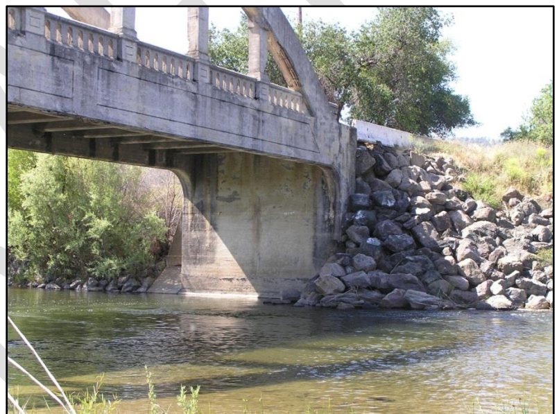
Abutment 1 left – RSP backfill after a storm event took out the bridge wingwall
