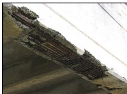
Tie Girder Spall – Pier 2 left isotropic view
