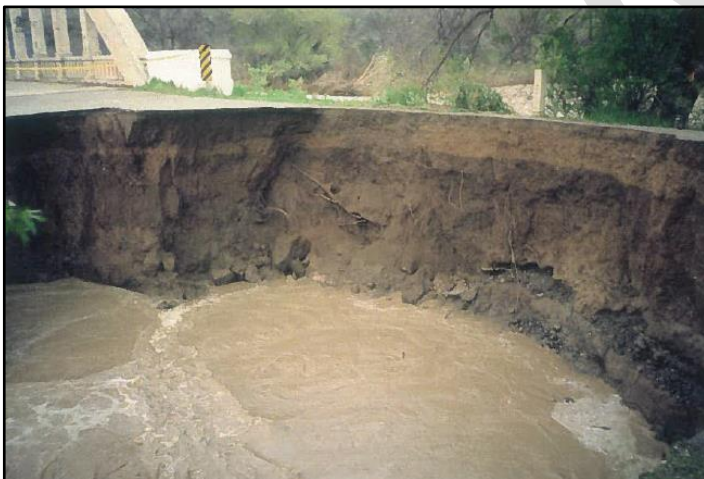
Storm Damage behind Abutment 1 in 1995
