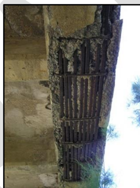
Tie Girder Spall – Pier 2 left looking from bottom
