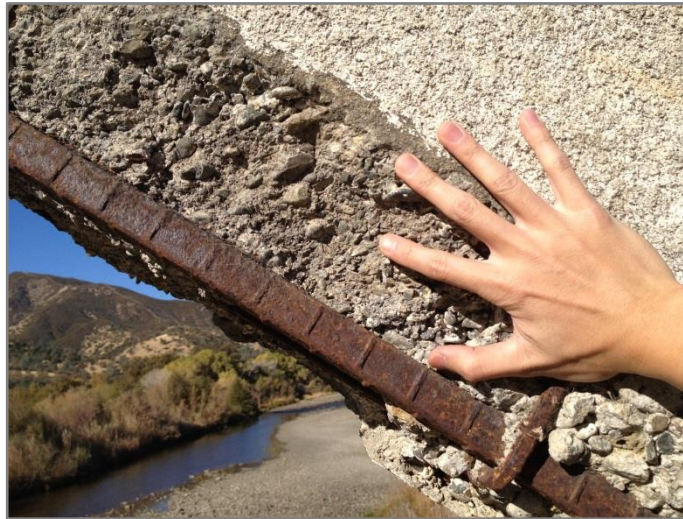
Extensive surface preparation is required for spalled surface area
