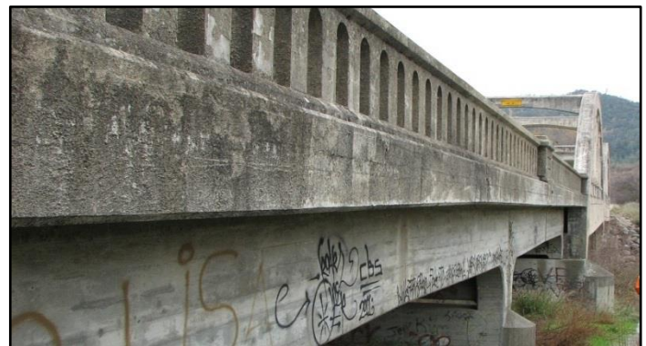
Rumsey Bridge Spans 3 and 4 – added in 1949 after flood damage to original bridge
