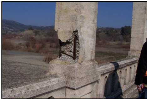
Severe Vertical Hanger Spalls
