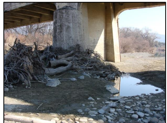
Debris built up Pier 2
