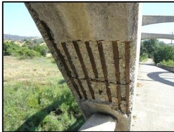
Arch Rib Spalls (Span 1 left arch, near Pier 2)
