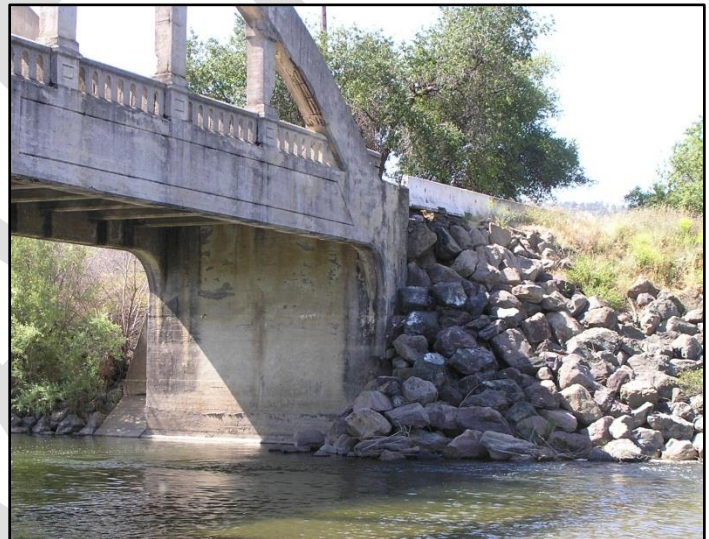
Abutment 1 Left wingwall washed out and backfilled with RSP
