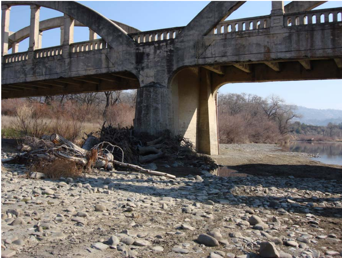
Figure 9: Debris buildup at Pier 2 (from 2007 field review)
