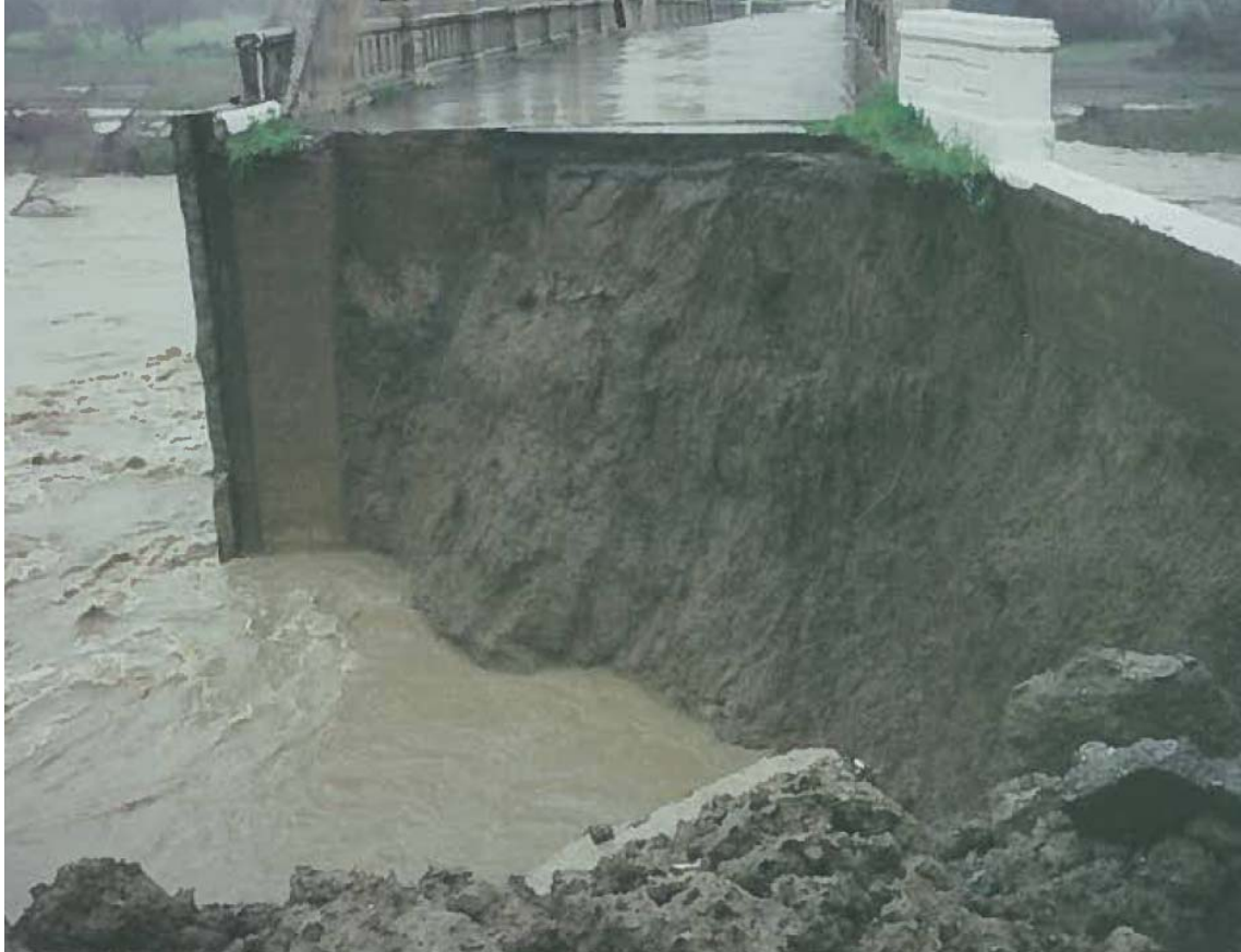
Figure 6: Erosion at Abutment during March 1995 storms (photo from QEI)
