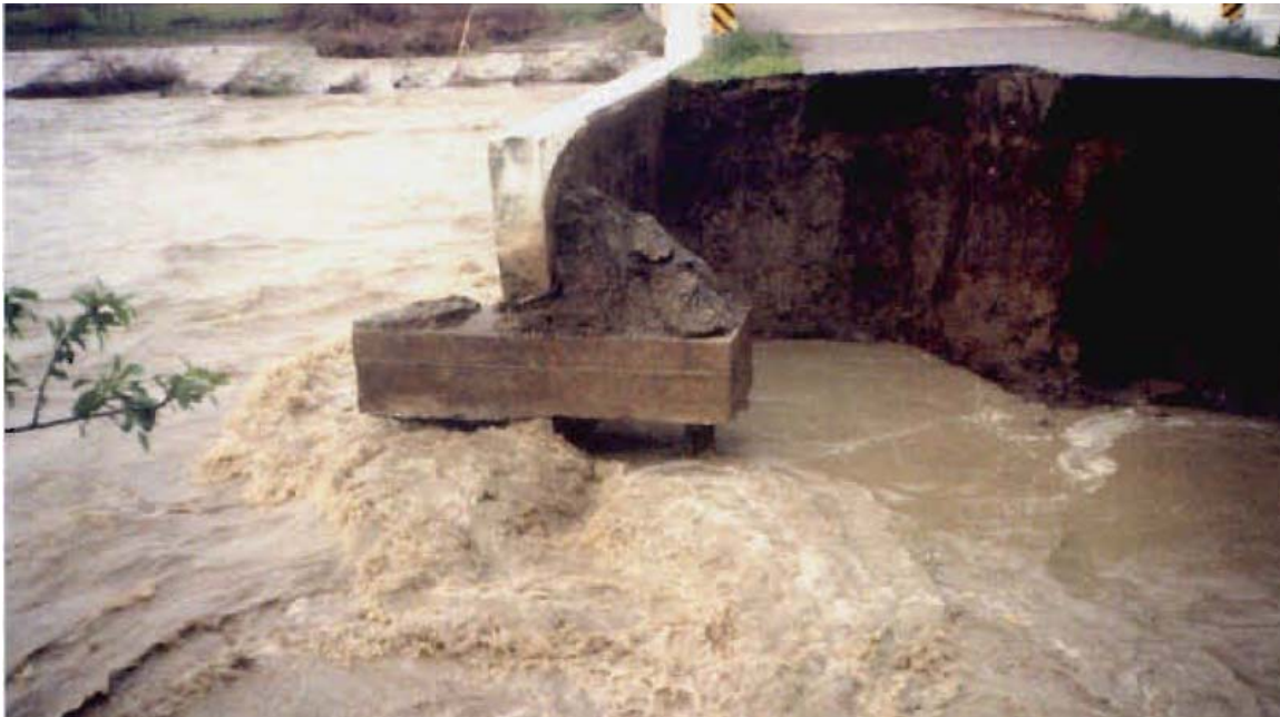
Figure 5: Wingwall prior to failure (from nbc, 1995)
