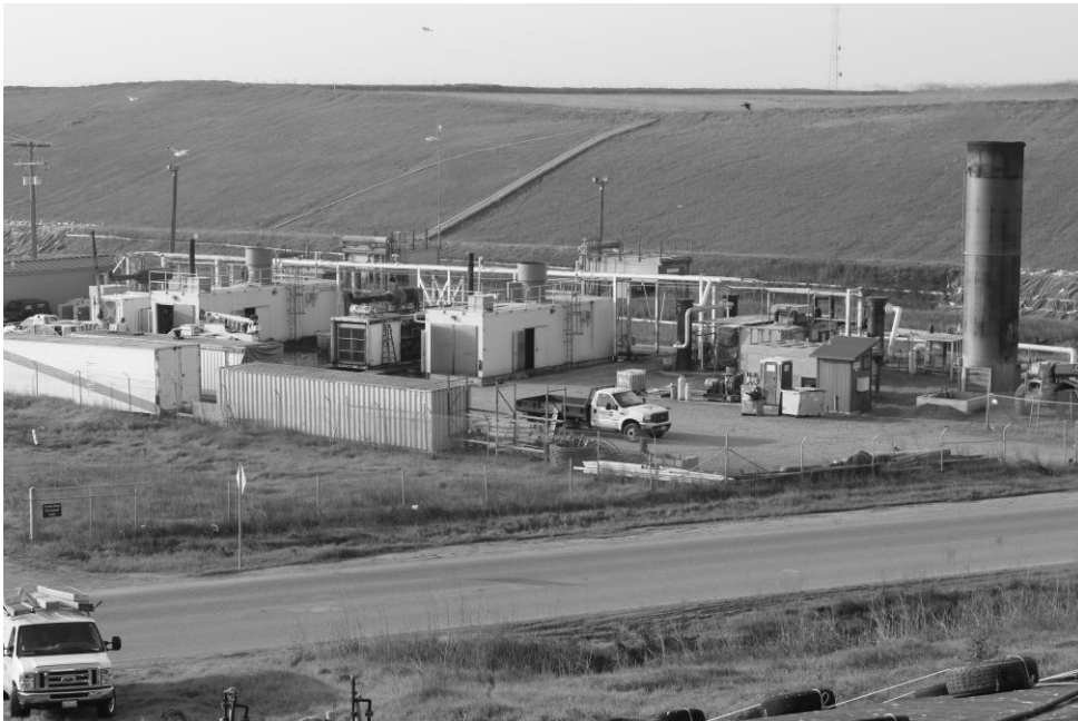
Figure 2: Yolo County Central Landfill methane gas-to-energy plant.
