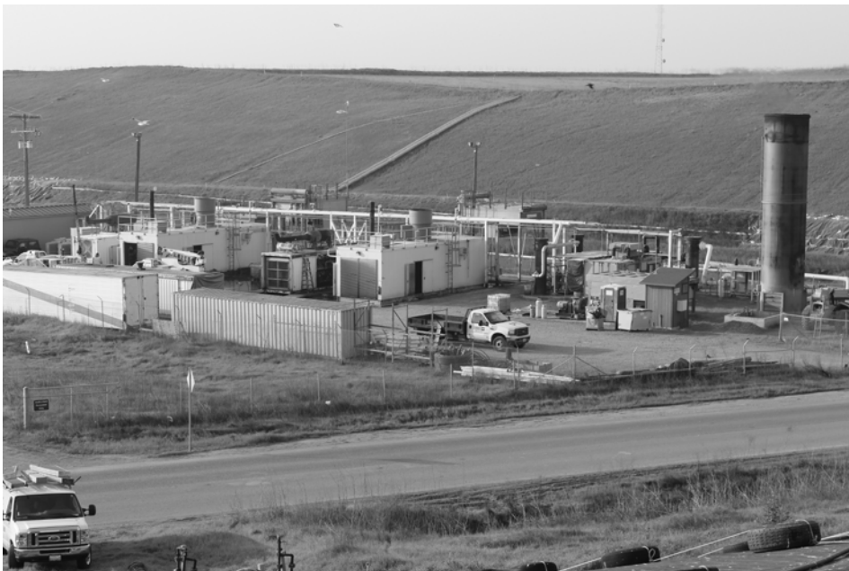
Figure 2: Yolo County Central Landfill methane gas-to-energy plant.
