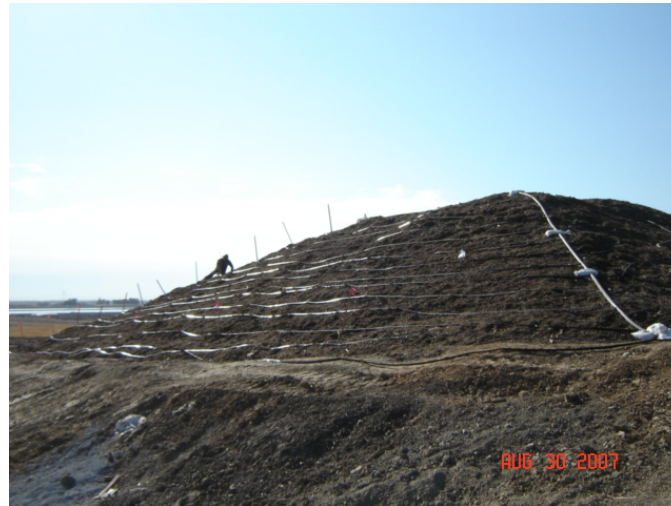
Picture 6: Drip irrigation system installed directly on waste
