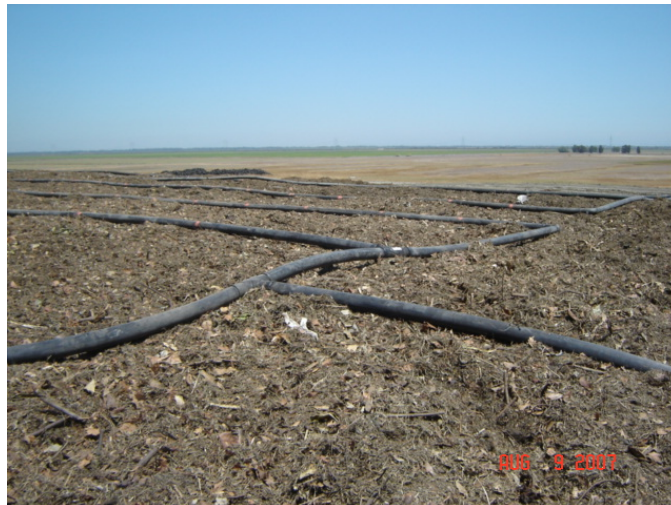
Picture 5: Horizontal liquid injection and recirculation system
