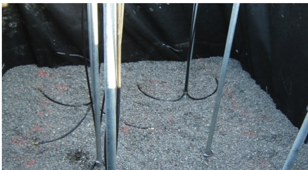
Figure 5. Overhead view of tubing used to distribute gas flow in base gravel layer.
