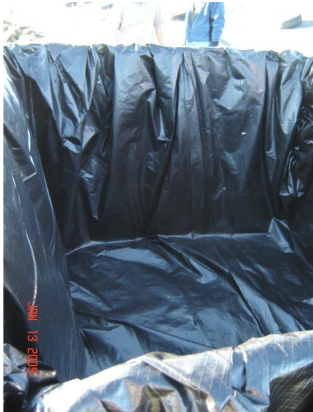
Figure 3. Interior of biocover cells lined with 8-mil reinforced polyethylene liner.
