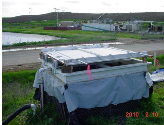
Figure 16. Biocover test cell with cover used for flux testing. The cover, propped up with pieces of wood in this photograph, is lowered onto the top of biocover and sealed during testing.
