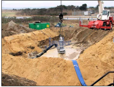
Dump Box with Pit
