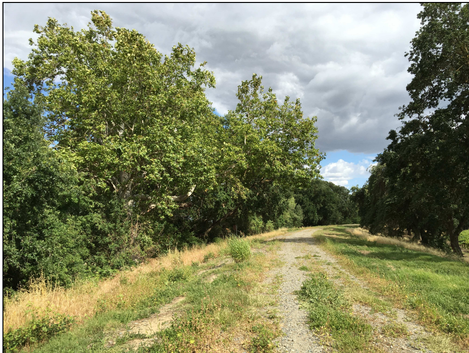
Plate 3. Elk Slough levee. Riparian along Elk Slough (valley oak and sycamore trees) is on left, valley oak trees at the outer toe of the levee is on the right.
