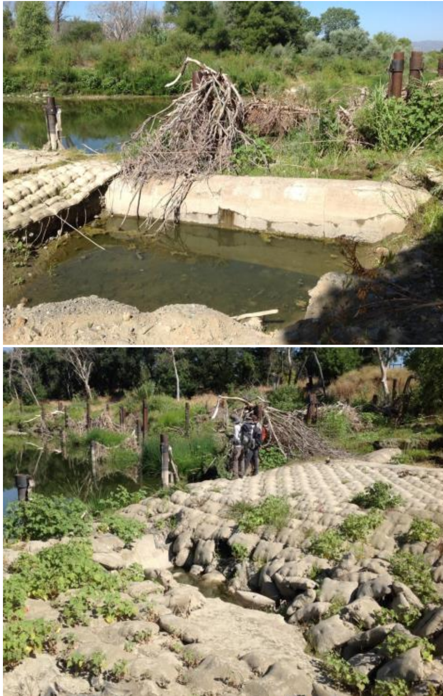
Figure 11: Photos showing scour holes in erosion control blanket at PG&E Palisades site.
