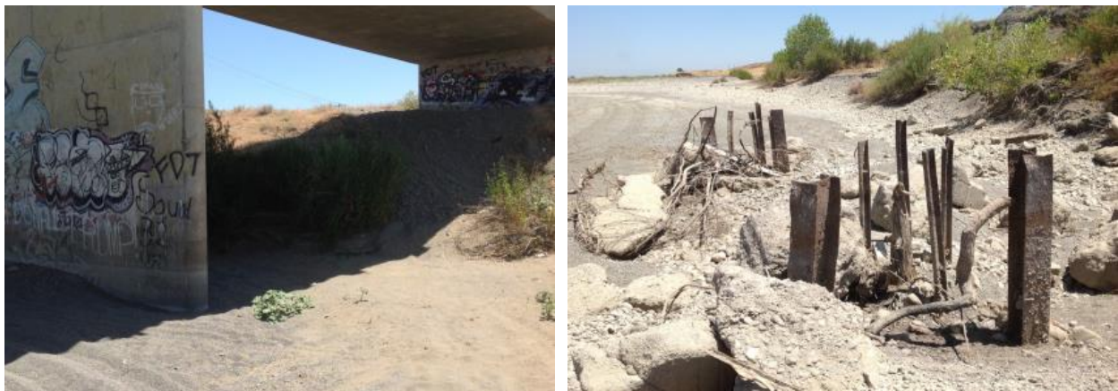
Figure 14: Photos showing un-scoured piers (left) and protruding steel piles immediately downstream of Esparto Bridge (right).
