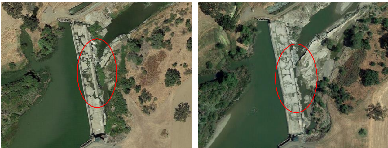
Figure 9: Photos showing Capay Dam in 2016 (left) and 2017 (right). 2017 photo shows several additional concrete pads were forced off the dam apron. Imagery courtesy of and copyright Google 2017.
