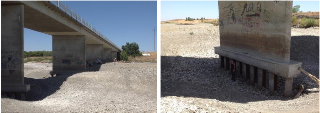
Figure 13: Photos showing undercut Esparto Bridge piers with member of County staff for scale (right photo).
