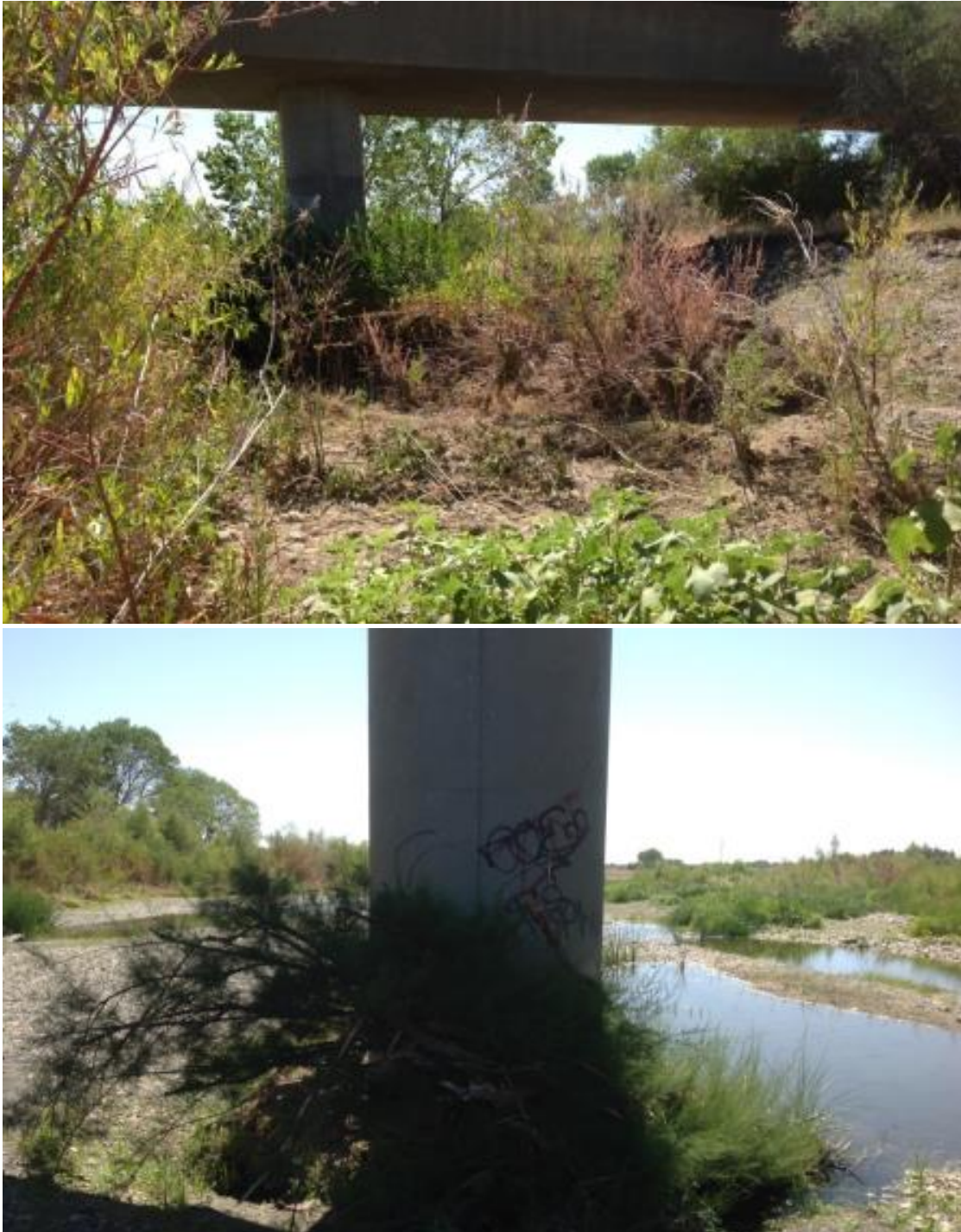
Figure 1: Photos showing Capay Bridge. The channel bed was not significantly scoured and vegetation in the bed is clearly visible.
