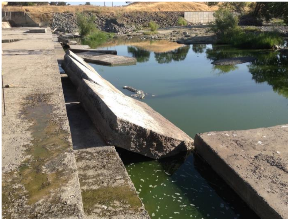
Figure 10: Photo showing concrete pads that have slid off the Capay Dam apron.
