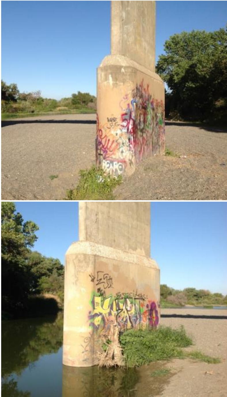
Figure 16: Photos showing Stephens Bridge piers with channel bed mostly bare after scouring.
