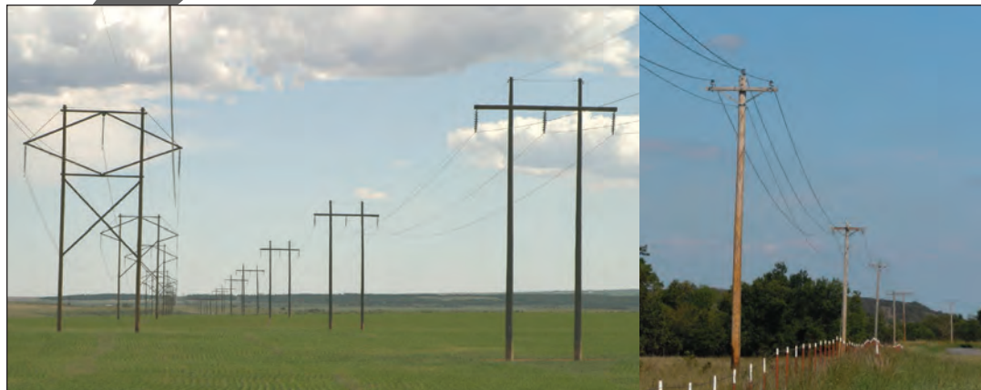
FIGURE 1.3: Transmission lines (left) and distribution lines (right).
