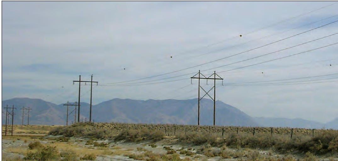
FIGURE 2.1: APLIC has helped fund studies on the effectiveness of different types of line marking devices in reducing bird collisions with power lines.
