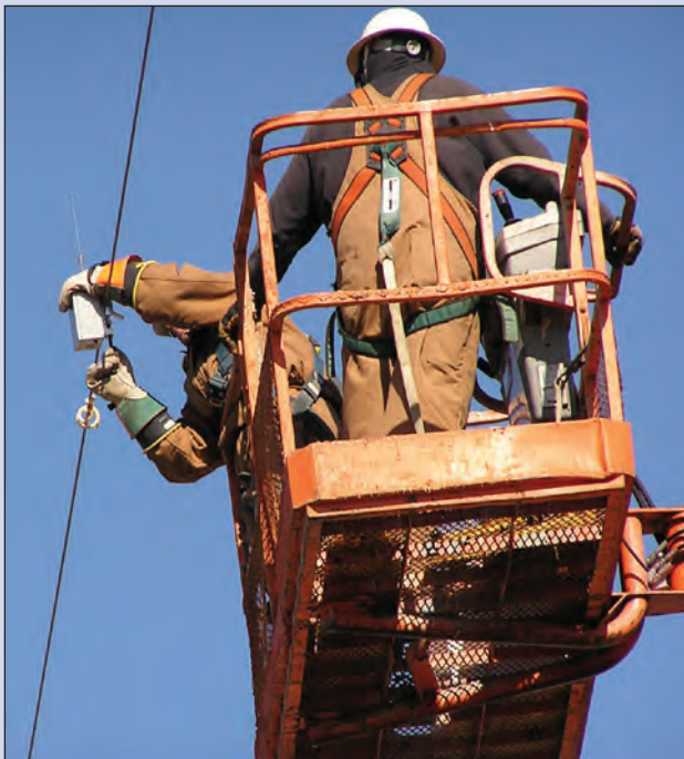
FIGURE 5.2: The Bird Strike Indicator, a tool used to detect bird strikes with power lines, can be installed from a bucket truck or helicopter.
