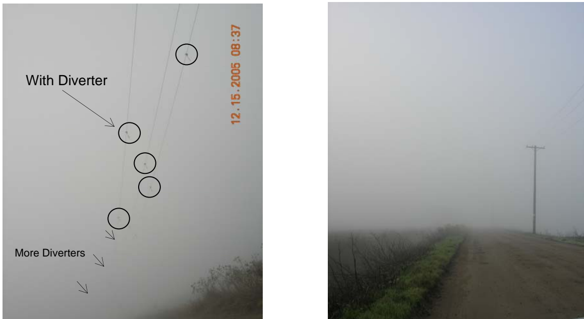
Figure 2. Distribution power lines at the study site (Staten Island, Walnut Grove, California). Heavy winter fog reduces visibility of distribution power lines with (left) and without (right) aerial marking devices. These devices, designed to increase line visibility, may not be effective in heavy fog.
