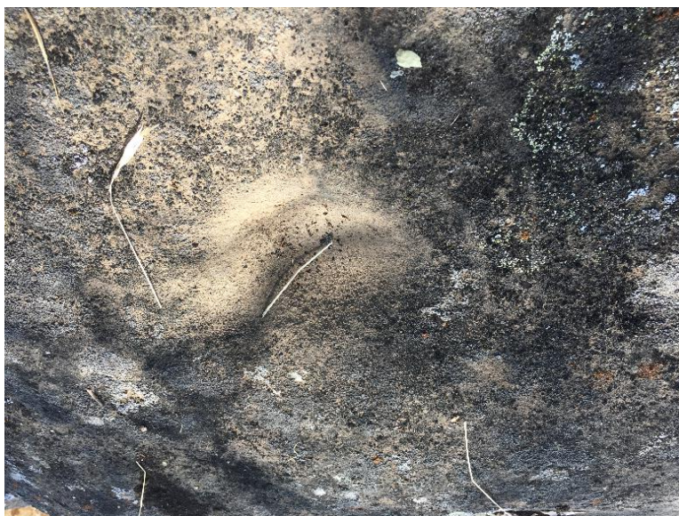
Photograph 17. MET Tower Location 2. KF-S-1, detail of Mortar Cup A. View facing down. A. Hallock. 10/11/2017.
