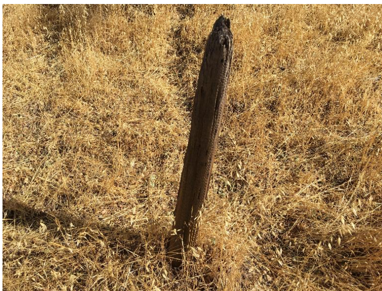
Photograph 28. MET Tower Location 3. Single deteriorated fence post. View facing down. A. Hallock. 10/11/2017.
