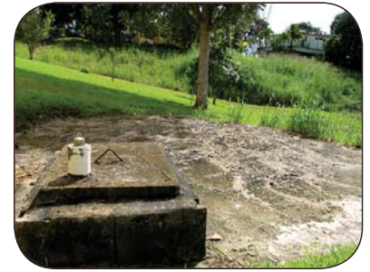
Keep septic tanks sealed.
