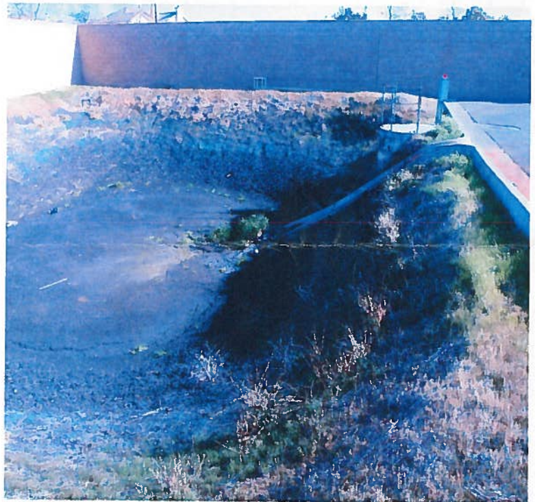
Figure 4. Storm water basin with solids from the WWTF.
