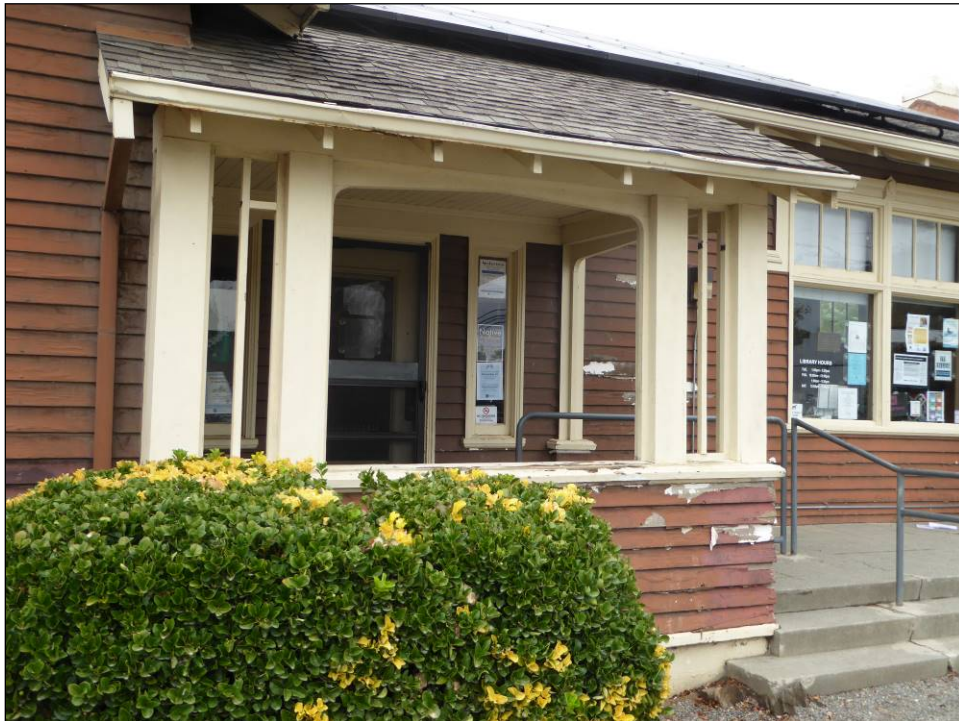
Figure 4-3. Top: Western gable end showing decorative half timbering and supporting bracket. Bottom: Front porch with supporting square pillars and flattened arch. Note rafter tails are visible under the roofline. Image source: JRP Historical Consulting.
