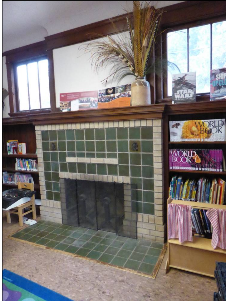
Photograph 5. Interior eastern end fireplace with green tile and cream brick. Flanking bookshelves are built in. Also visible is the high picture rail and cove ceiling.
