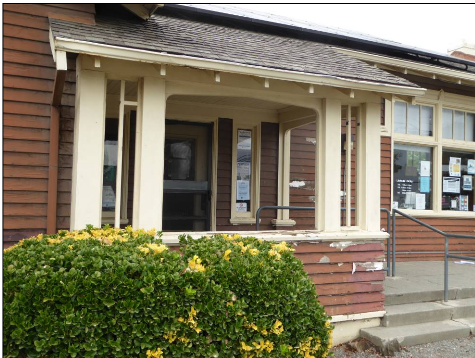
Photograph 4. Front porch with supporting square pillars and flattened arch. Rafter tails are visible under the roofline.
