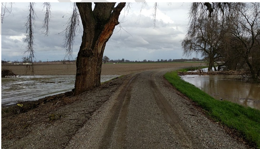
Figure 8: Seepage during February 2019 High Water Event
