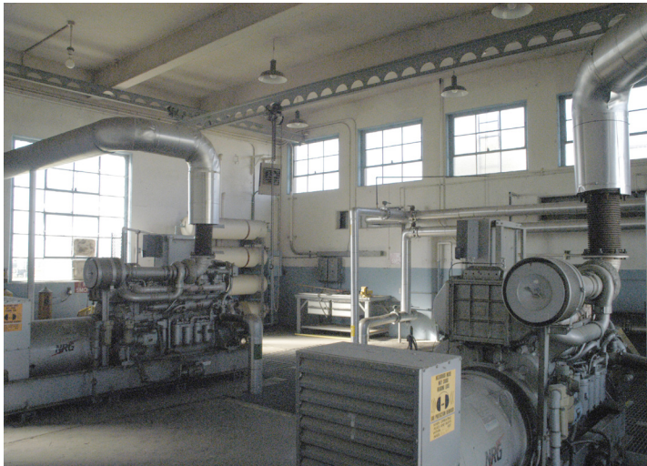
(b) Main Generator Room
