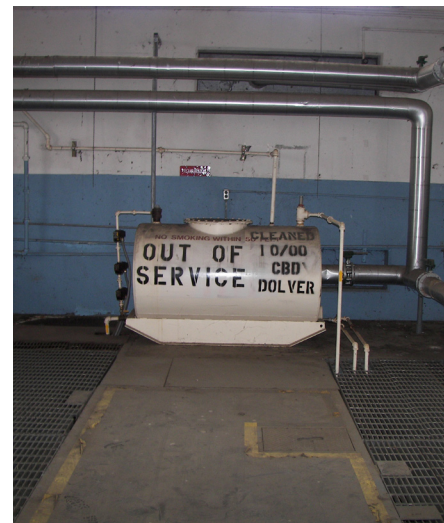
250,000 Gallon Diesel Tank in Generator Room
