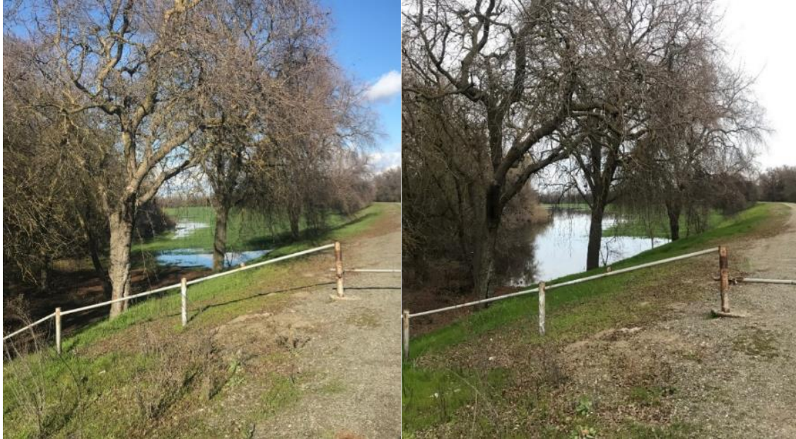
Figure 5 Seepage along Sacramento River at levee mile 4.0, February 19, 2019 & March 1, 2019
