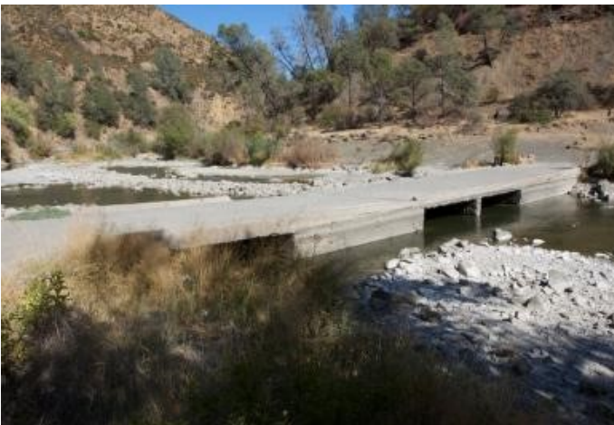
$3M in state funding was secured to replace the Low Water Bridge at County Road 40
