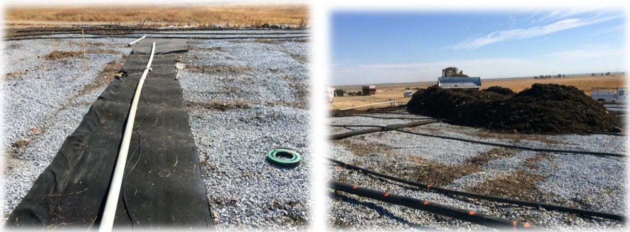
Figure 4. Temperature and pressure tubing installed for Cell monitoring and leachate injection/recirculation and gas collection piping were installed.
