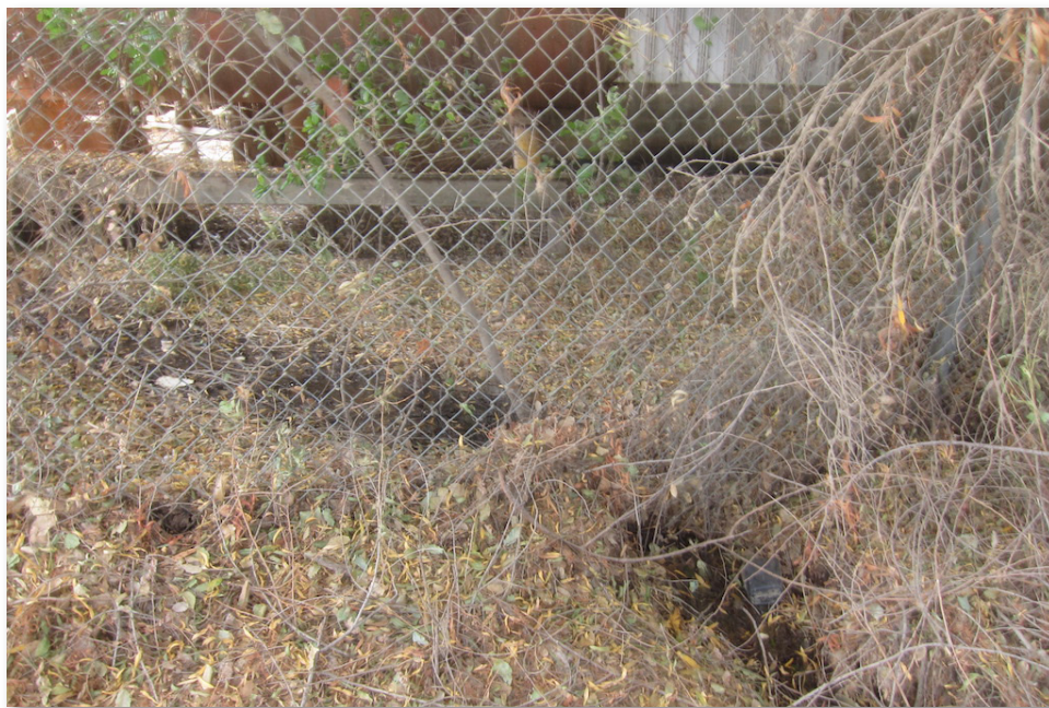
Photo 4. Leakage flow entering site under property boundary fence.
