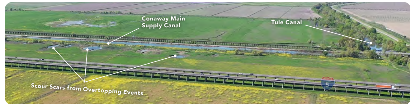
View of Conaway Main Supply Canal, looking north. Photo by Conaway Ranch.
