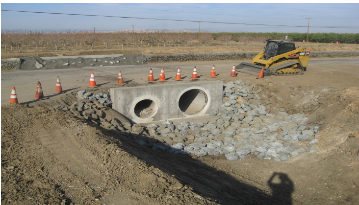
Construction work underway as part of the Madison Flood Protection Improvement Plan.
