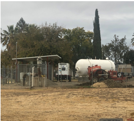
Generators in Madison were purchased to ensure water/wastewater operations during power outages.
