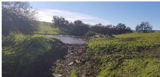
Photo 8: Earthen dam failure at stock pond adjacent to project area. Taken facing southwest.
