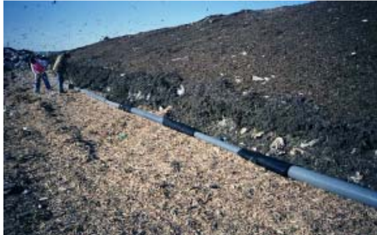
Image 3-2. Horizontal LFG collection line
