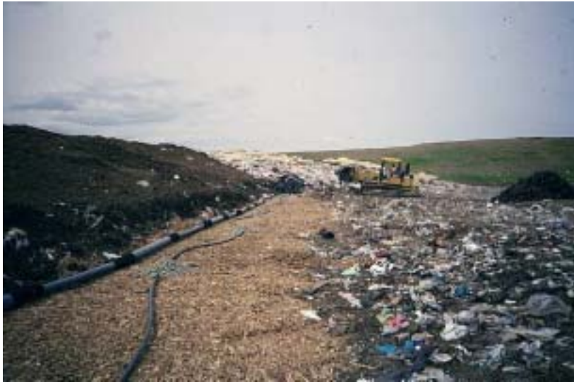
Image 3-1. Horizontal LFG and leachate injection lines installed and being covered by shredded tires.
