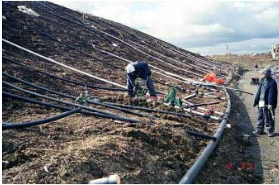
Image 5-5. Aerobic leachate injection header and lateral
