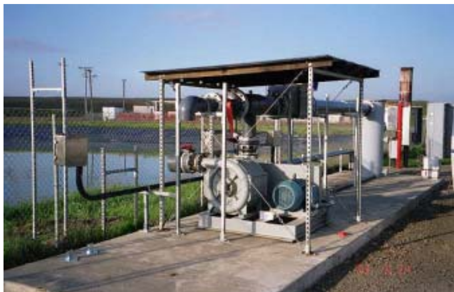
Image 5-7: Aerobic Cell Blower Station
