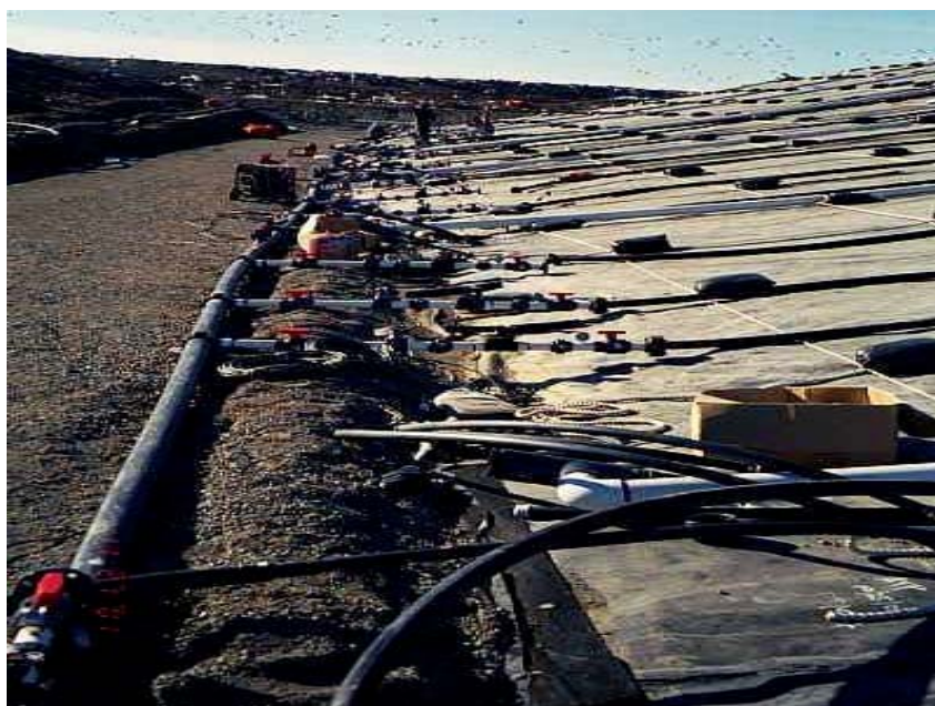
Image 3-7. Leachate injection header and laterals
