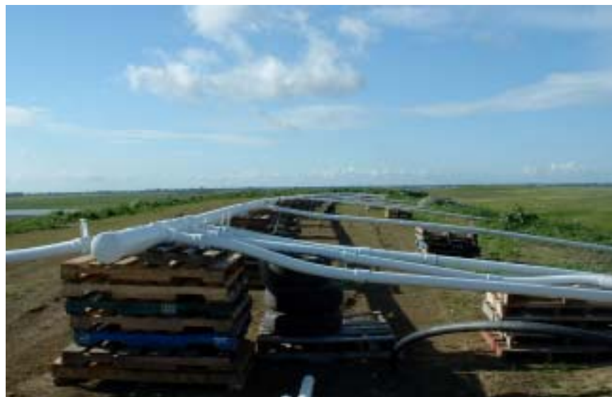
Image 4-3. LFG collection laterals connected to the main header line located on top the cell.
