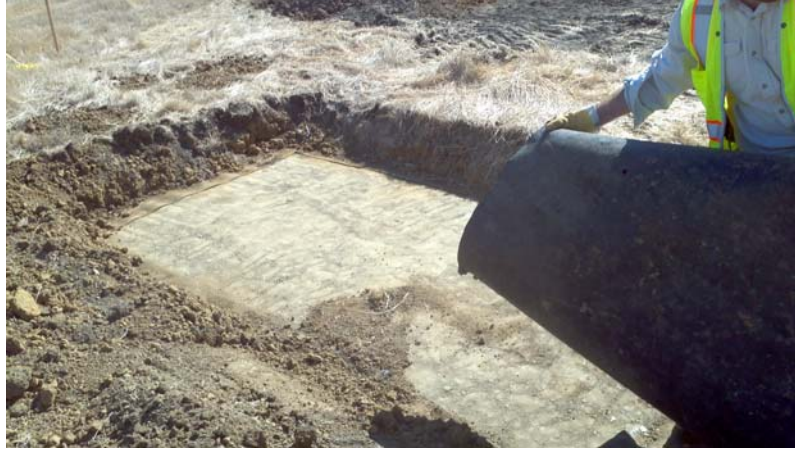
Figure 3: Soil removed over the liner and area ready for excavation of cover soil below liner.
