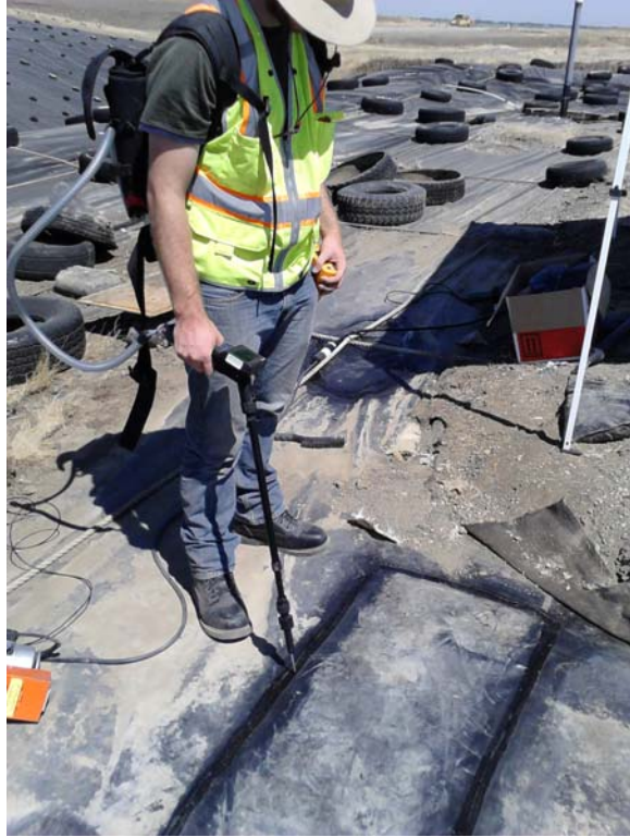
Figure 7: Repaired liner is scanned for methane leaks prior to placement of cover soil over liner.
