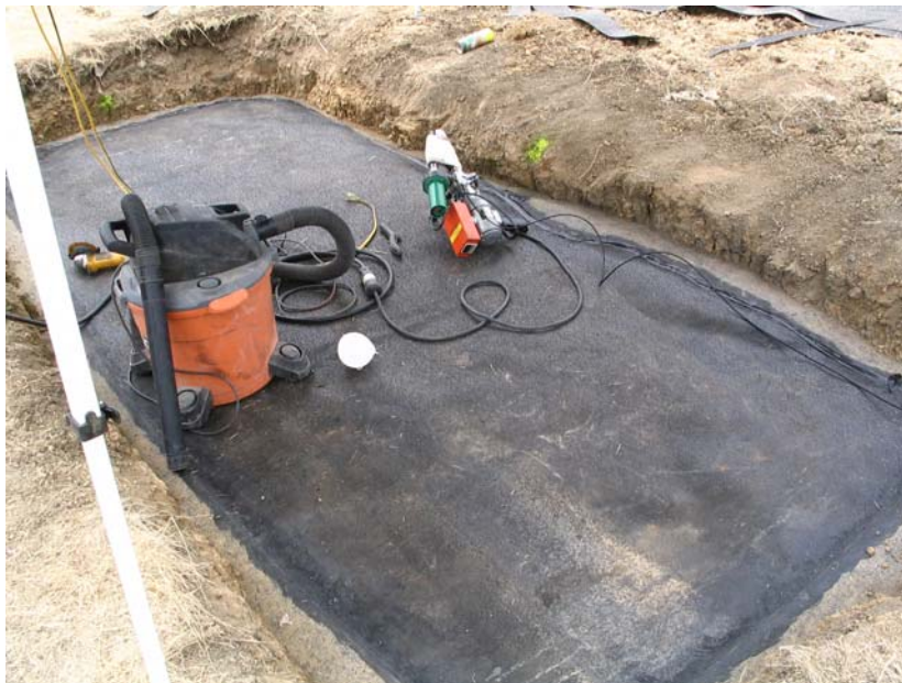
Figure 8: Completely repaired liner prior to placement of cover soil and returned back to original condition.
