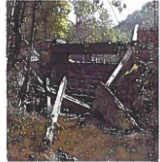
Damaged historic dam
