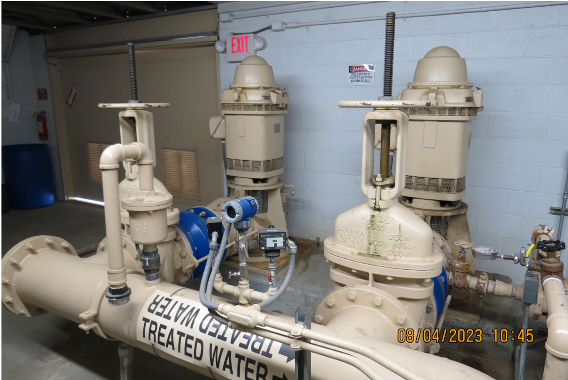
Replace Booster Pumps
