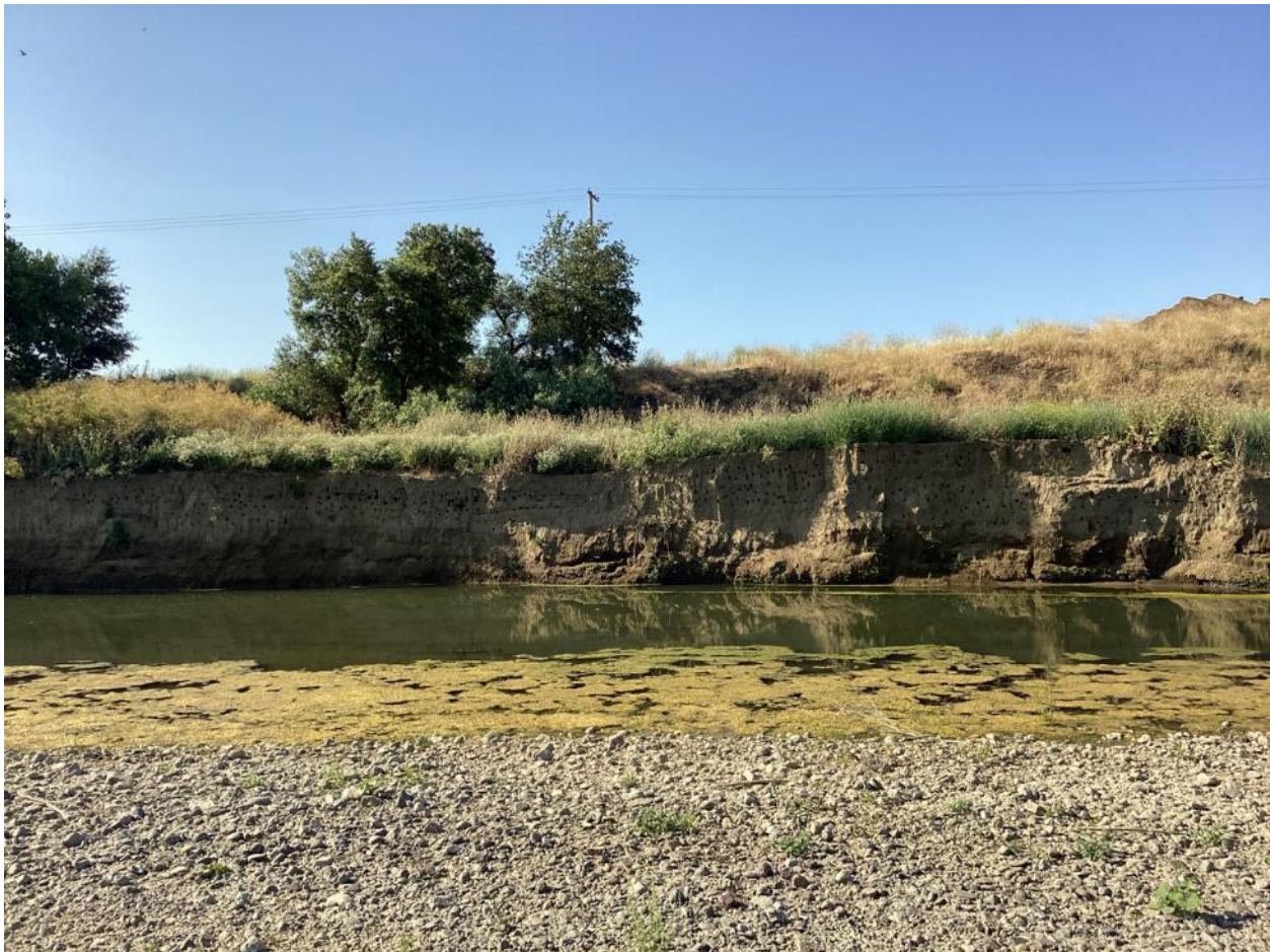
Figure 2-26. Apparently new bank erosion and bank swallow activity. (2023)
