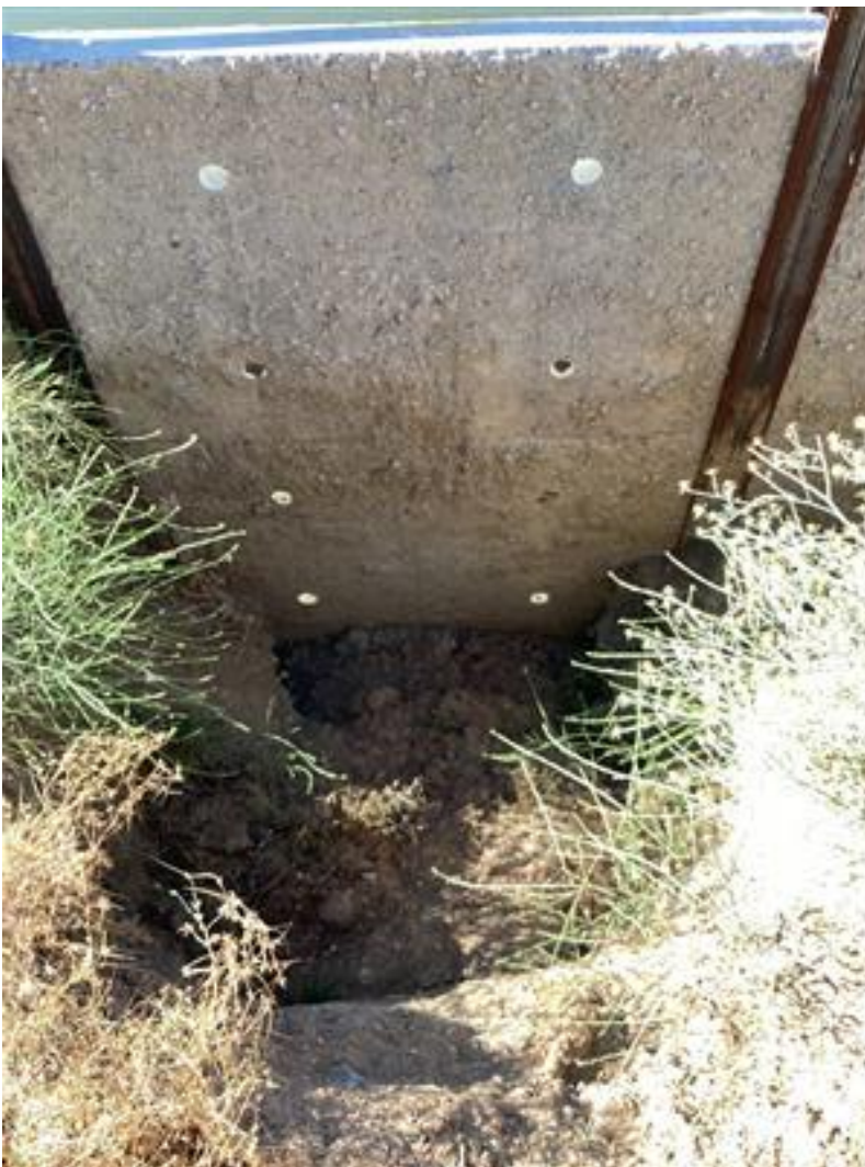
Figure 2-14. View of soil erosion behind Bank Repair Wall at Capay Dam. (2023)
