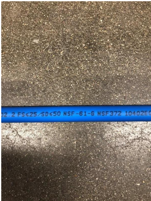
Blue potable PEX line with NSF label
