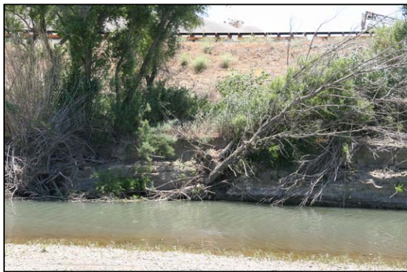
Figure 50. Meander undercuts the levee at RM 20.45.
