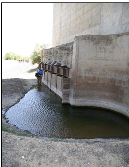
Figure 46: Scour along support vane under I-505 Bridge.
