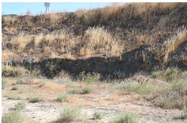
Figure 35: Erosion at the levee toe, RM 23.2.
