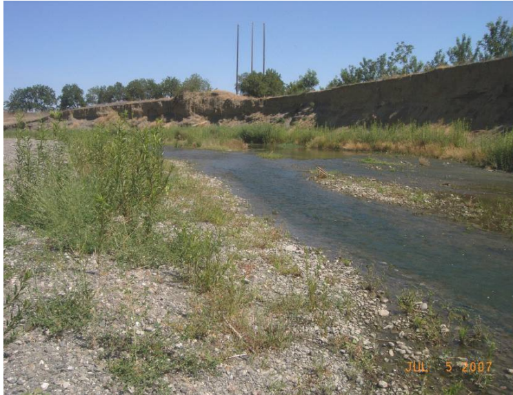
Figure 41. Bank erosion at the outside bend of the meander at the Scheuring property.
