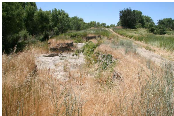
Figure 78: Eroded berm separates Correll pit from Cache Creek at RM 13.7.
