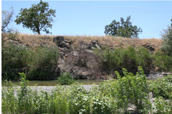
Figure 53: Low, oversteepened bank with loose blocks at RM 19.4.
