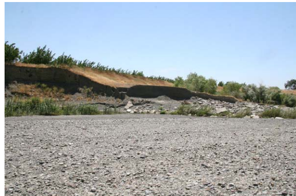
Figure 43: Active erosion of upstream spur dike, RM 21.55 north bank.
