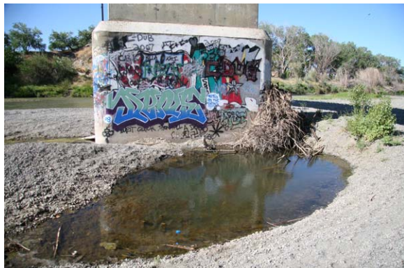
Figure 71: Scour pool under CR-94B Bridge.
