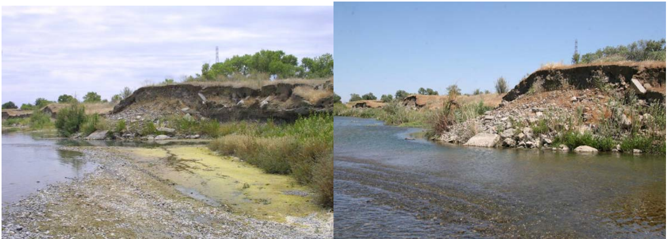
Figure 58 and 59. Eroded spur dikes at RM 18.6, south bank in 2007 (left) and 2008 (right).
