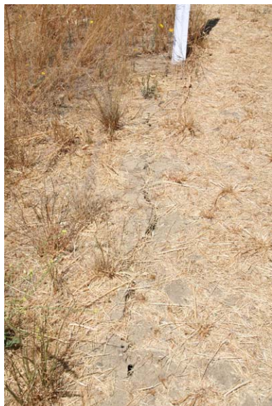
Figure 88: Cracks in soil at the edge of the road (Huff's Corner) show that the south bank is unstable.
