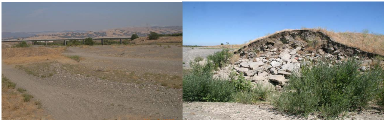
Figure 30 (left) and 31 (right). At RM 24, Sediment deposition between Syar spur dikes and scour at toe of spur dikes.
