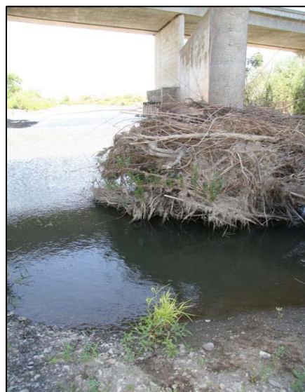
Figure 47: Scour hole on upstream end of I-505 Bridge support.
