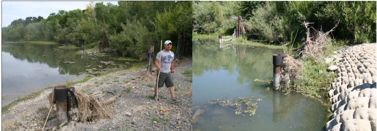
Figure 10. Prior to 2008 (left photo), sediment had been effectively trapped at the steel piles and nets next to the concrete pillow blanket. In 2008 (right photo), this sediment had been eroded away.
