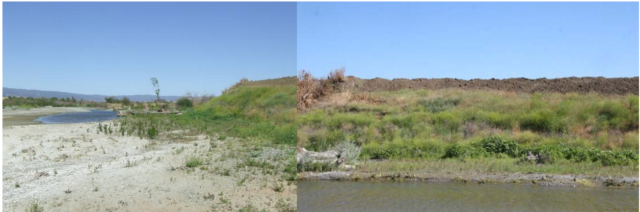
Figure 38 (left) and 39 (right). Teichert bank protection with scour behind root wads and loose soil on top of levee.
