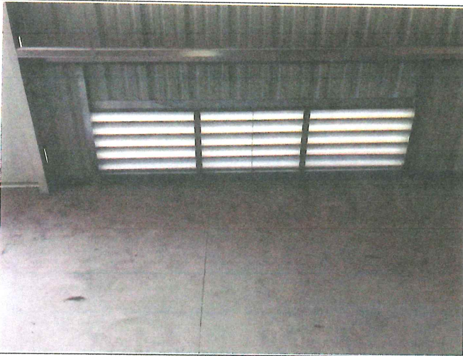
Photo One Caption TYPICAL VENT (TAKEN 08/08/2017)
