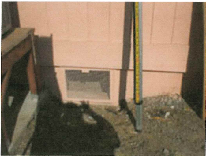
April 24, 2008 Large Vent in Rear
