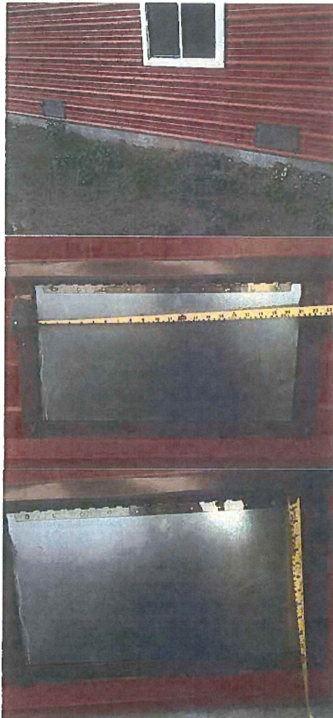
FLOOD VENTS ALONG PERIMETER 02/19/14
