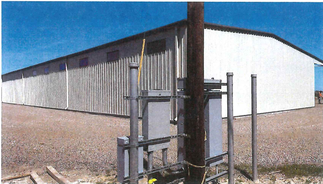
Photo Two Caption: REAR VIEW (TAKEN 04/10/2024)
